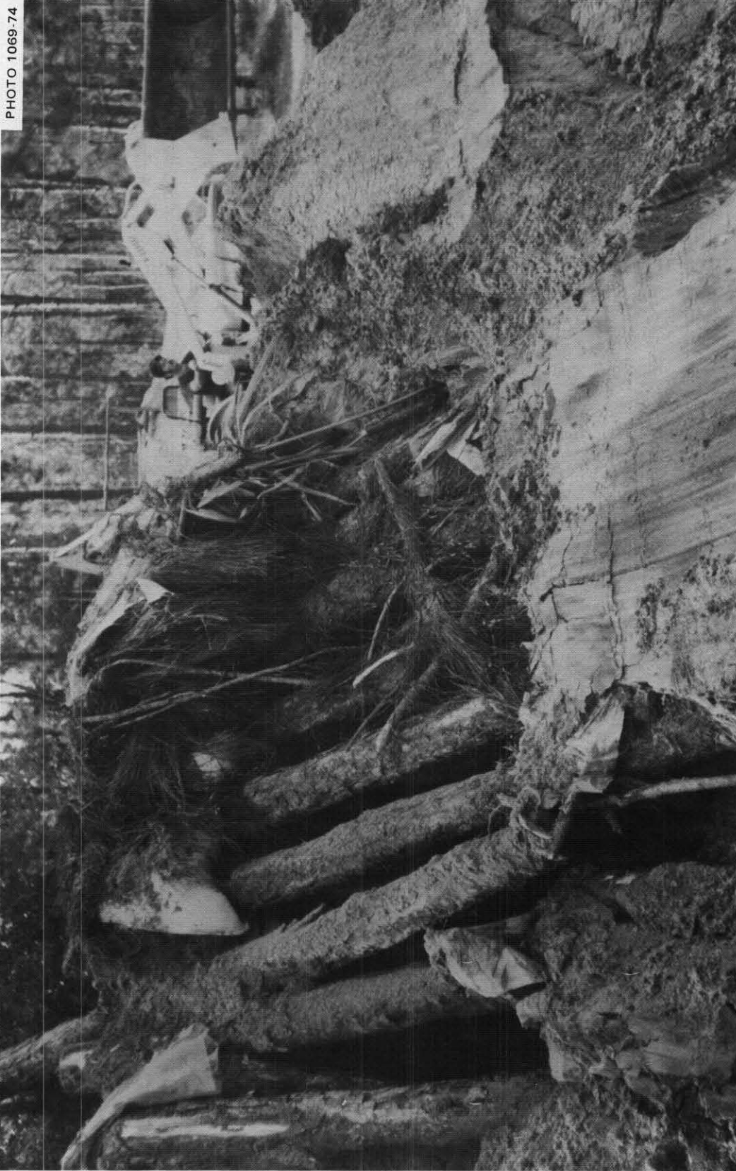
Fig. 5.40. View after a backhoe had started to demolish the Waldens' Ridge-Pole Shelter, which proved to be decidedly sturdy. Note that some of the wall poles were broken before they were moved off the ridge poles, or the ridge pole had been moved significantly.
